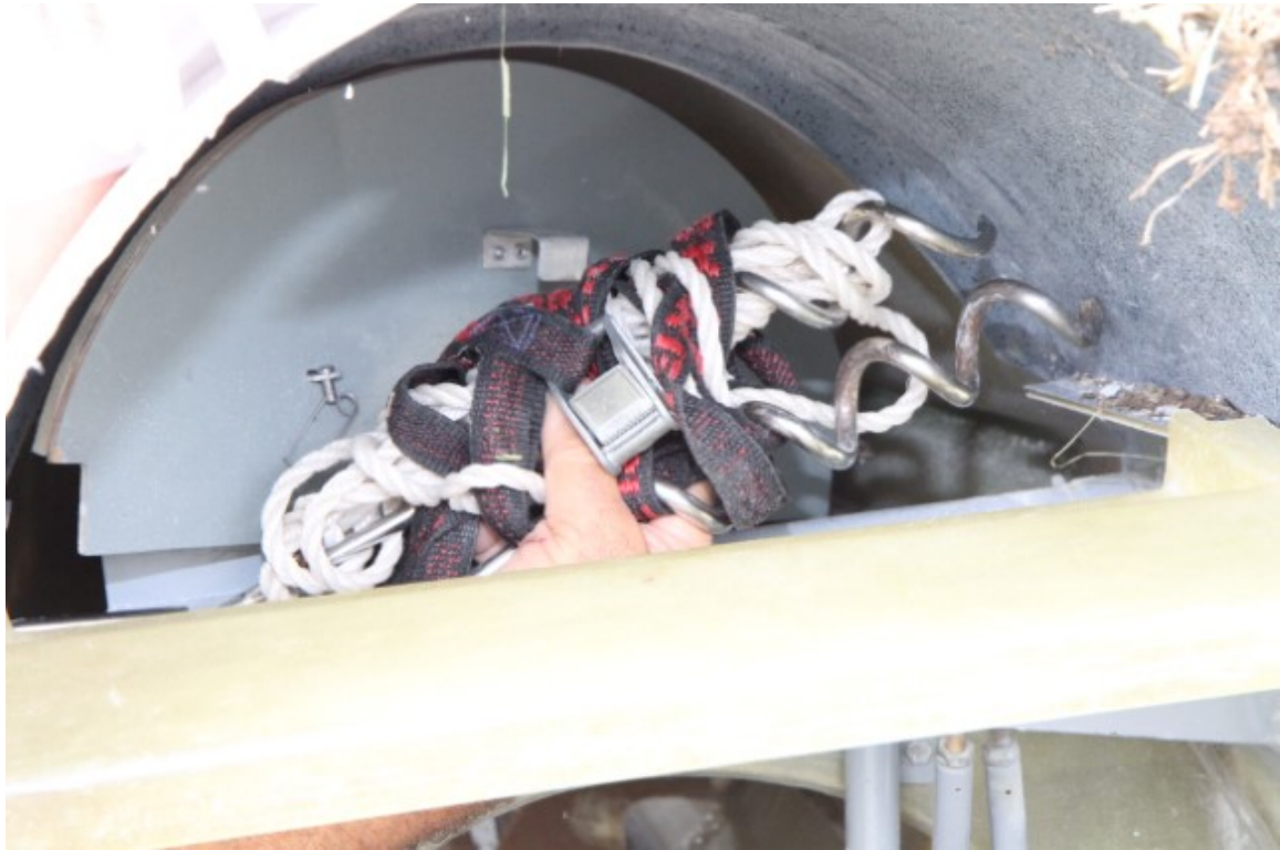
Demonstration of the gap between the stowage tray and the aft bulkhead which is difficult to detect when looking aft.
