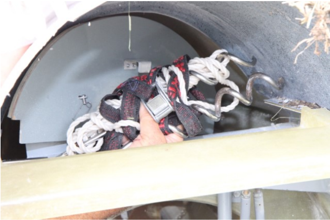
Demonstration of the gap between the stowage tray and the aft bulkhead which is difficult to detect when looking aft.
