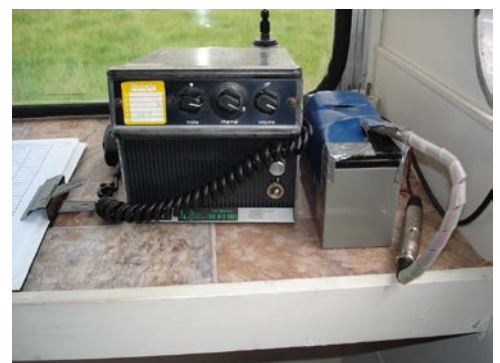
A typical base radio set-up
